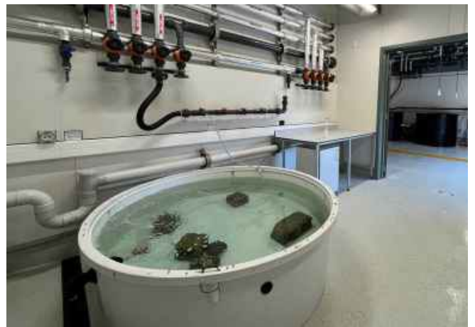
Inside one of the five temperature controlled seawater rooms in the new facility.
